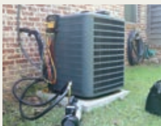
Pre-season HVAC tune ups
